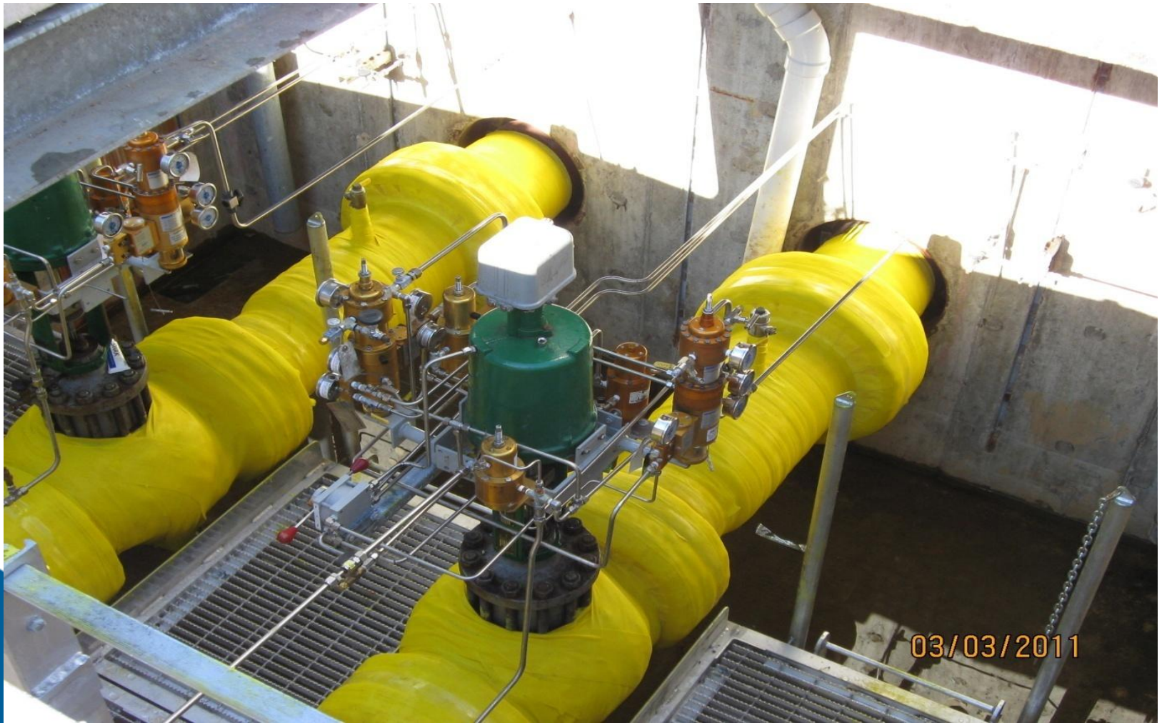
Pair of pneumatically operated 24 inch valves at MAOP 1440 psig
